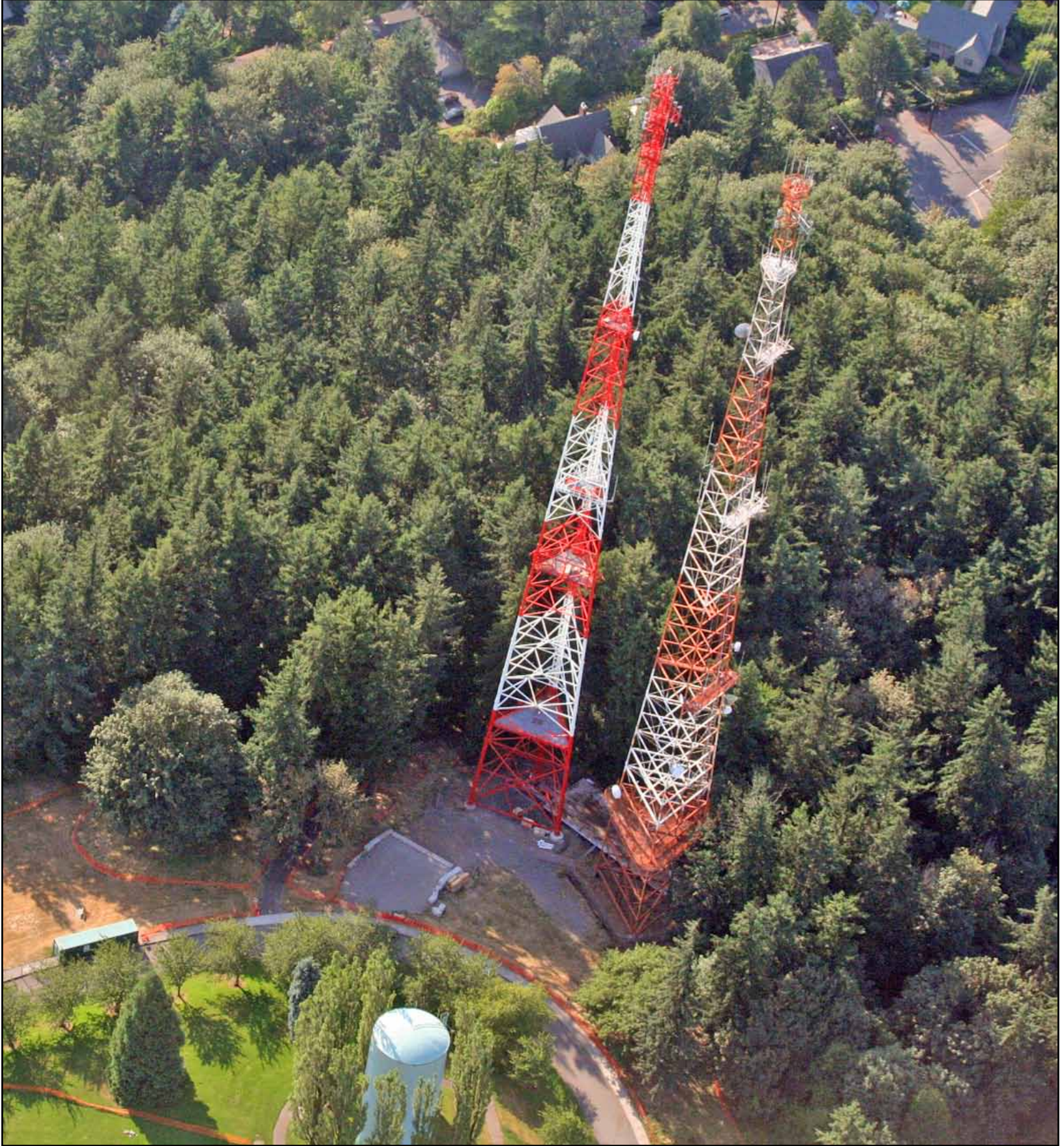
Antennas are being removed from the old Council Crest tower on the right. Dismantling of the old tower will begin soon. The replacement tower on the left takes over transmission of public safety radio communications for police, firefighters, and other public safety personnel.
