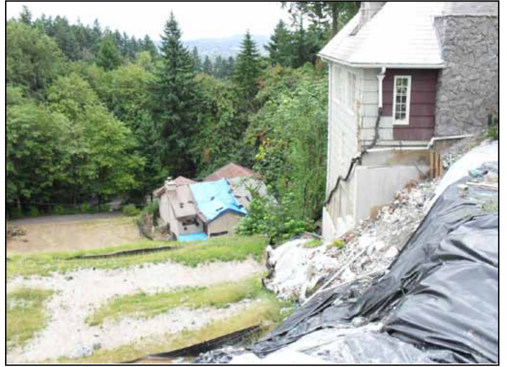
Damage from October 2008 slide
