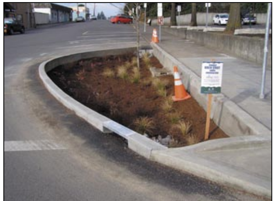
The new curb extension and vegetated swale in front of Key Bank. The swale will pick up water from both SW Troy and 35th. Later this spring, similar facilities are planned for construction in front of Starbucks and in SW 32nd next to Lucky Lab.
